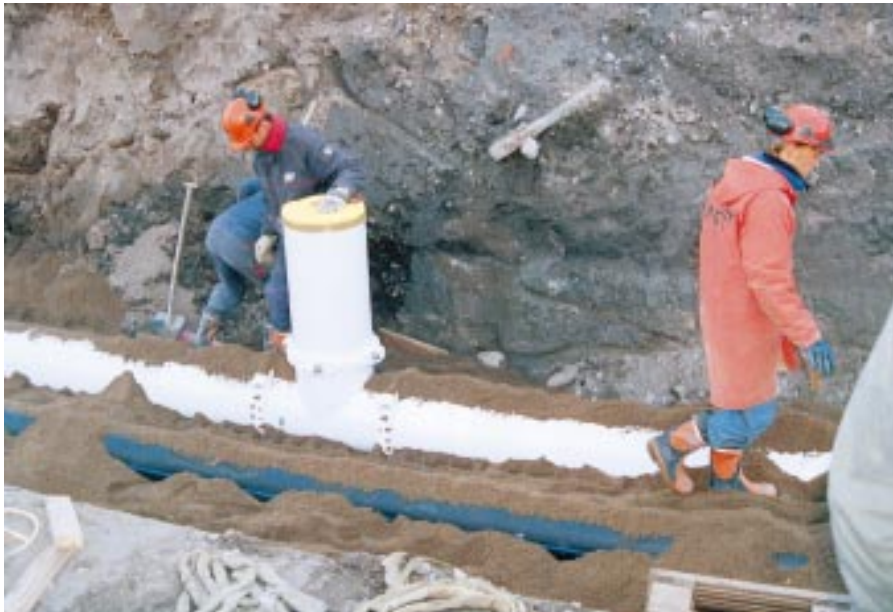
The 330 meter sewage pipeline will at a malfunction be exposed to the aggressive and very corrosive sewage water from the boiler. Alvenius TP-pipes are proven to be suitable for this type of application.
